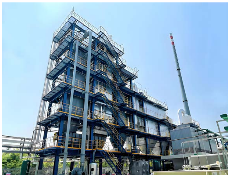
Waste Liquid and Wastewater Incineration System with Supporting Flue Gas Treatment Facilities
