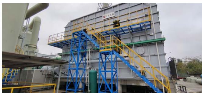
New High-efficiency Intelligent RTO System
